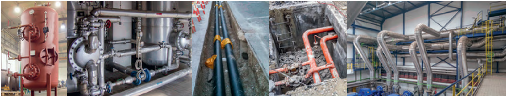
District heating systems (Osijek, Sisak, Zagreb)
